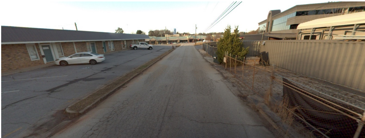
Figure 3.6: Very Poor PCI
