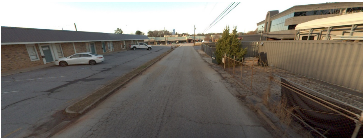
Figure 4.6: Very Poor PCI
