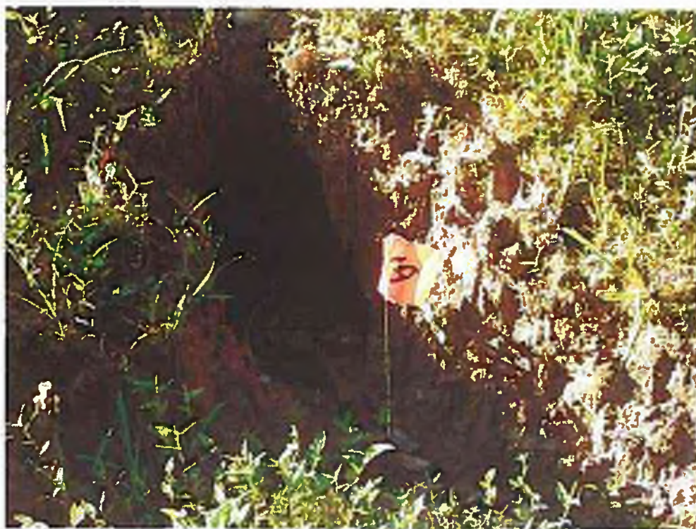
Erosional Hole at Base of Smaller Slough
