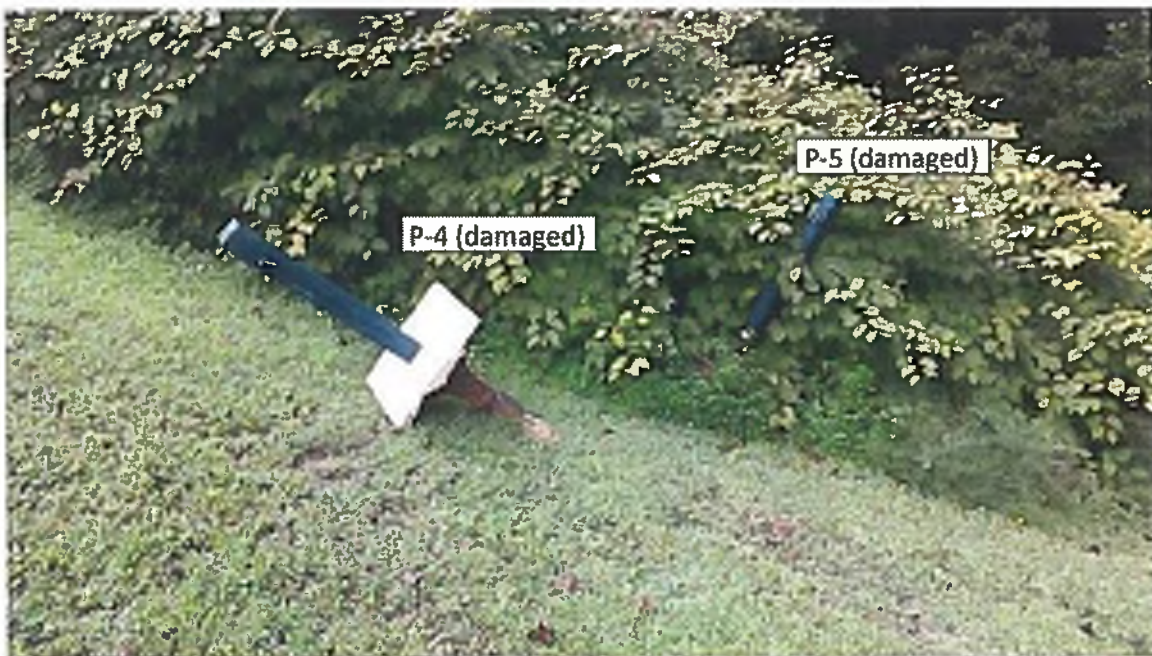
Damaged Piezometers P-4 and P-5; Facing West; 09/08/2014
