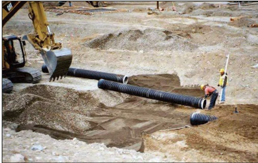
Figure 53. —Installation of profile wall corrugated pipe for a drainpipe replacement during a modification of an embankment dam.
