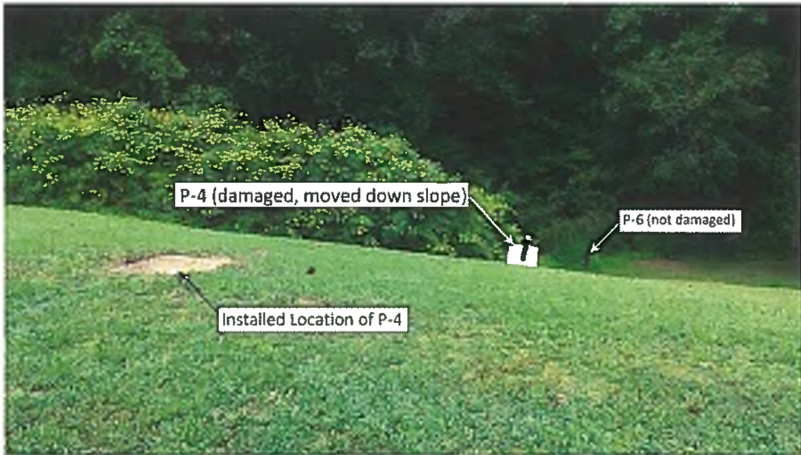
Piezometers P-4 through P-6; Facing Northwest; 09/08/2014
