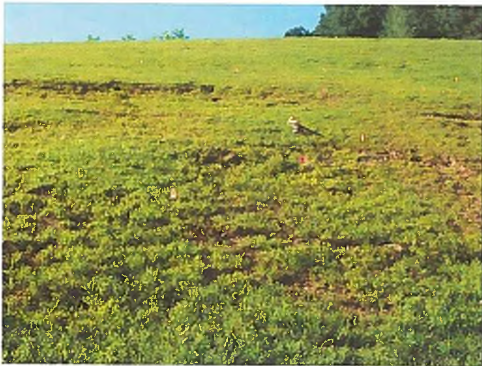
Larger Slough Area – Downstream Slope, Erin Lake Dam
