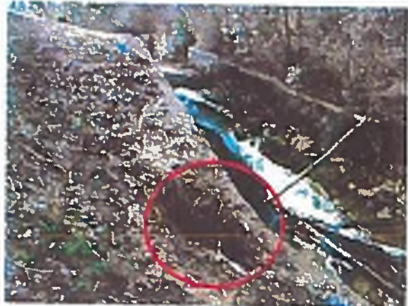
Hole at the right wing-wall of emergency spillway
