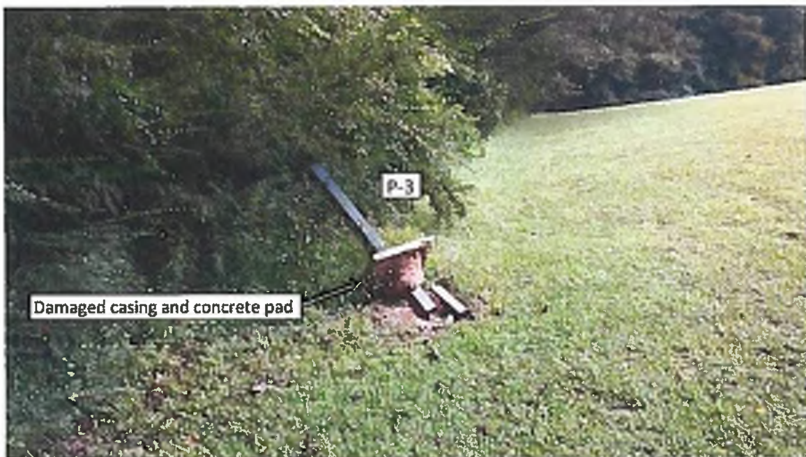
Damaged Piezometer P-3; Facing East; 09/08/2014
