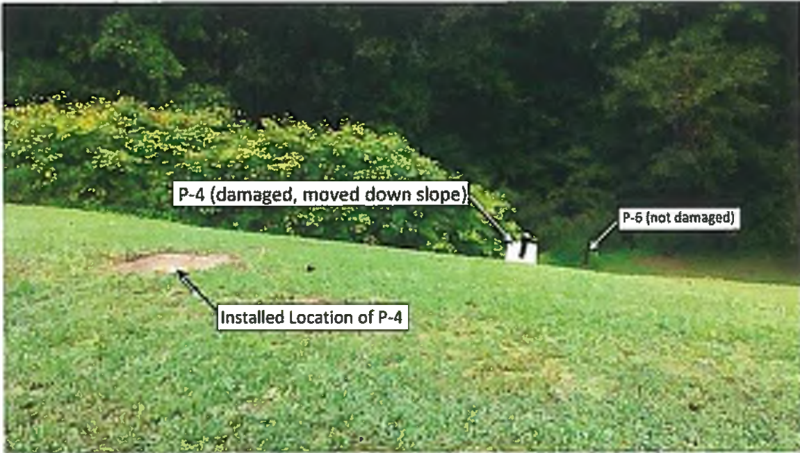
Piezometers P-4 through P-6; Facing Northwest; 09/08/2014
