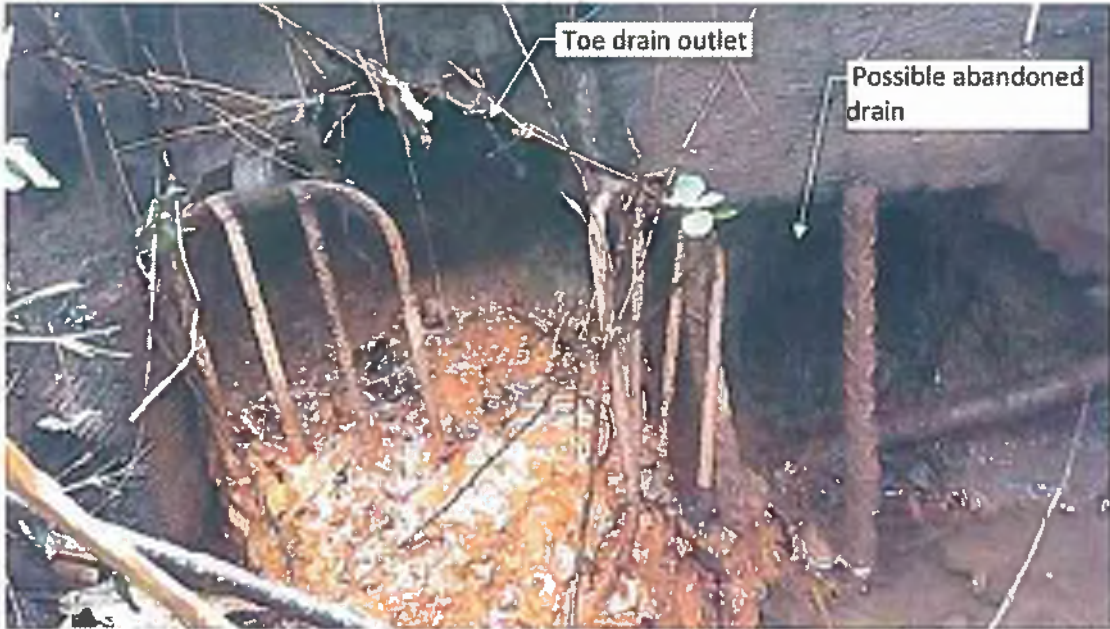
Toe drain outlet (left) and possible abandoned drain (right); photographed on 1/10/2014
