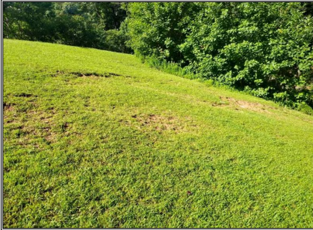
Site conditions showing the wooded area of the downstream of the dam.
