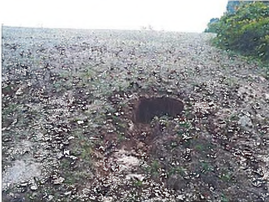
Erosion hole; photographed on 10/28/2013
