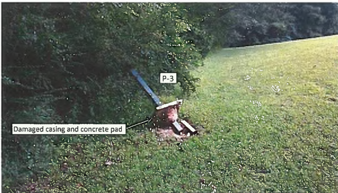
Damaged Piezometer P-3; Facing East; 09/08/2014
