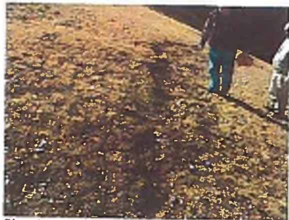
Slough on the downstream slope (mid-section)
