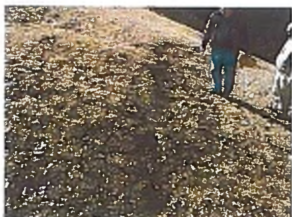
Slough on the downstream slope (mid-section)
