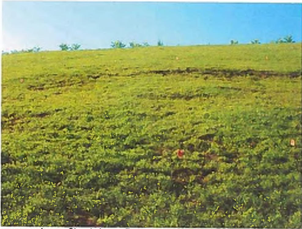
Larger Slough Area – Downstream Slope, Erin Lake Dam
