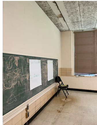
Roof leaks in building
