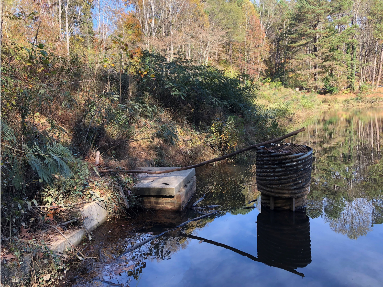
Outlet Control Structure
