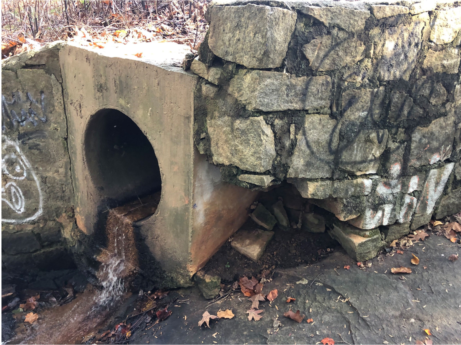
Downstream Outlet Pipe
